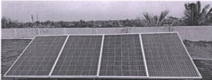
Fig 4.1 Solar PV plant
