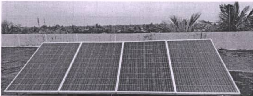
Fig 5.1 Solar PV plant
