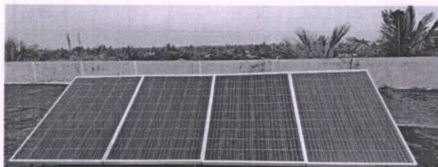
Fig 5.1 Solar PV plant
