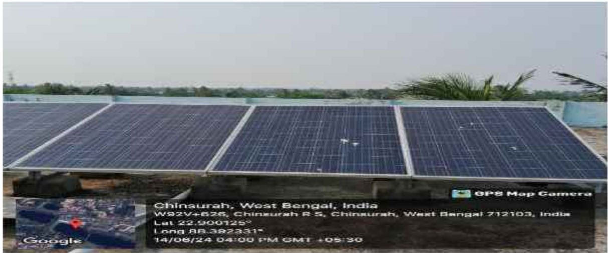
SOLAR PANEL ON THE ROOF OF SECURITY BLOCK
