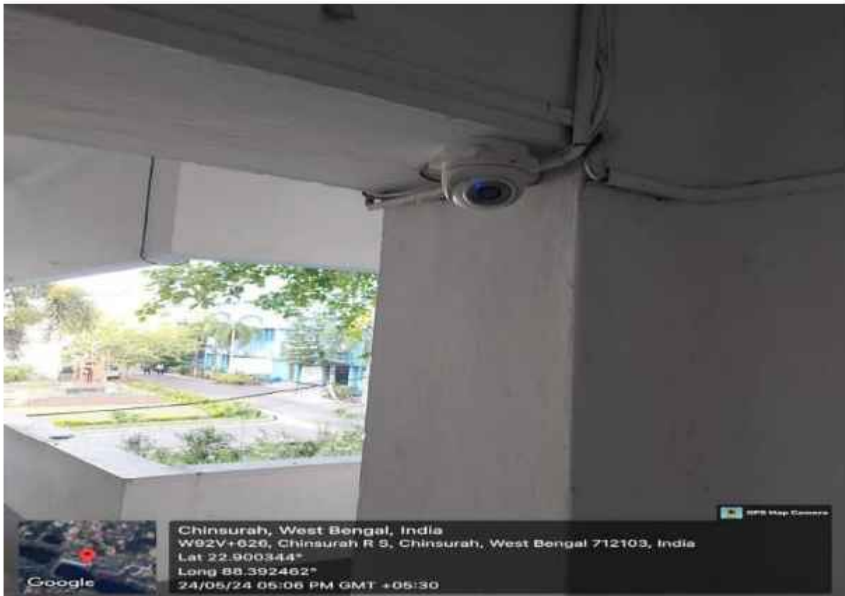
CCTV: Within College Building
