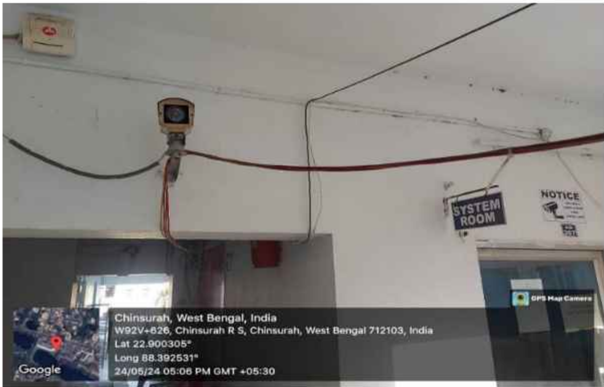
CCTV: Within College Building
