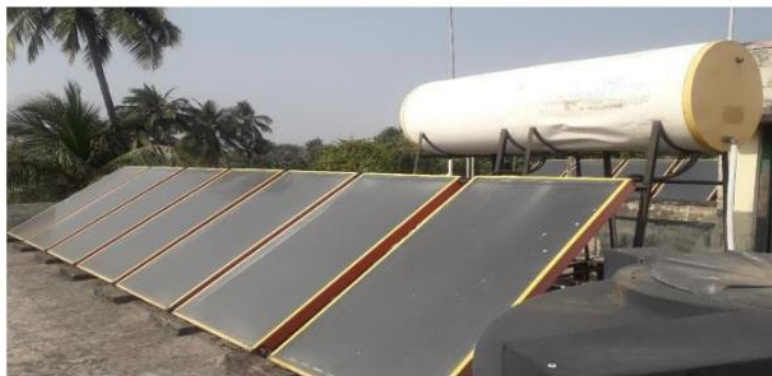
SOLAR THERMAL SYSTEM TO GENERATE HOT WATER
