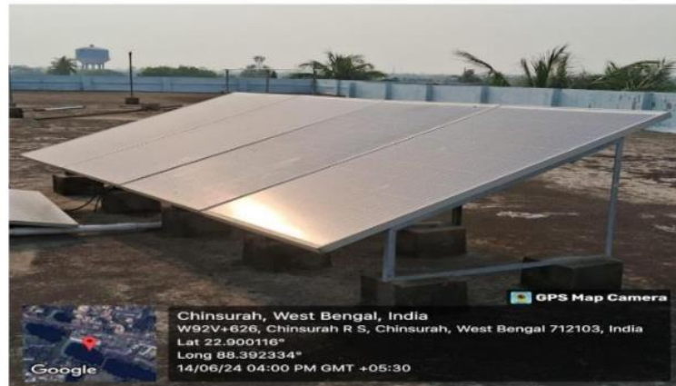
SOLAR PANEL ON THE ROOF OF THE FACULTY BLOCK
