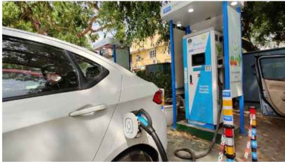
Fig:1 Charging Station
